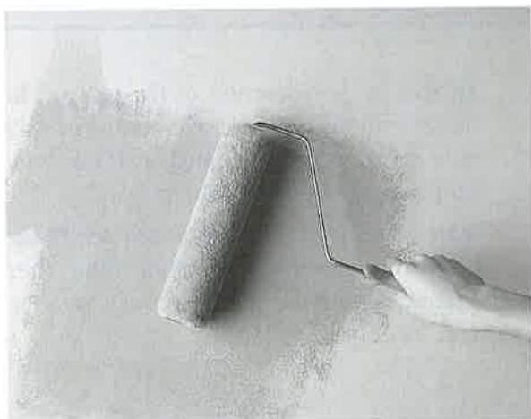
Fig. 33-5 —For large areas, you can use a small roller to apply the paint. Then use light brush strokes to feather it out.
